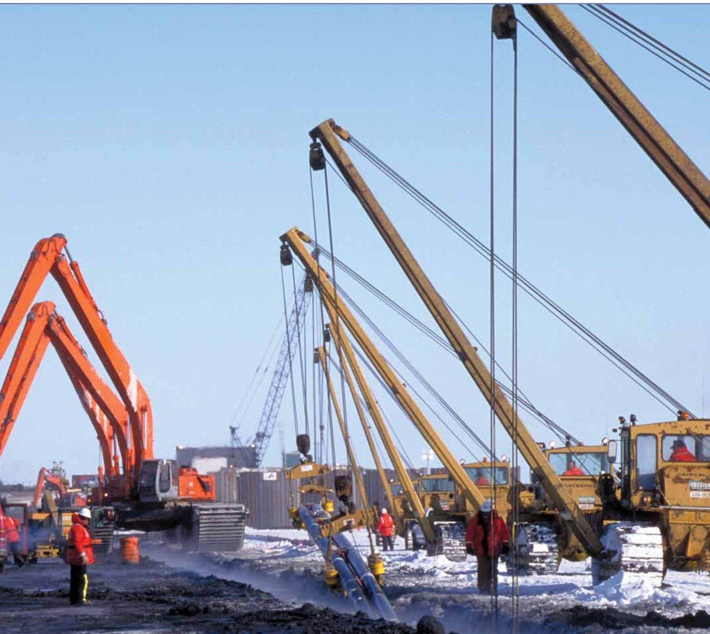
Cranes lower pipes into a trench between two ice platforms on the Caspian Sea Photo courtesy of AIC Canada
